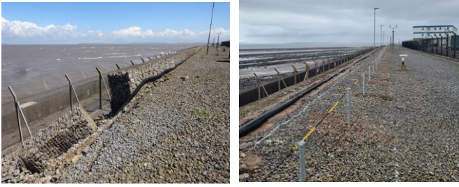
Fig. 5 A section of the Gabion Wall to the north perimeter of the site had partially collapsed. Work to stabilise the wall included the removal of the top baskets with excavation behind the wall as a relief.
