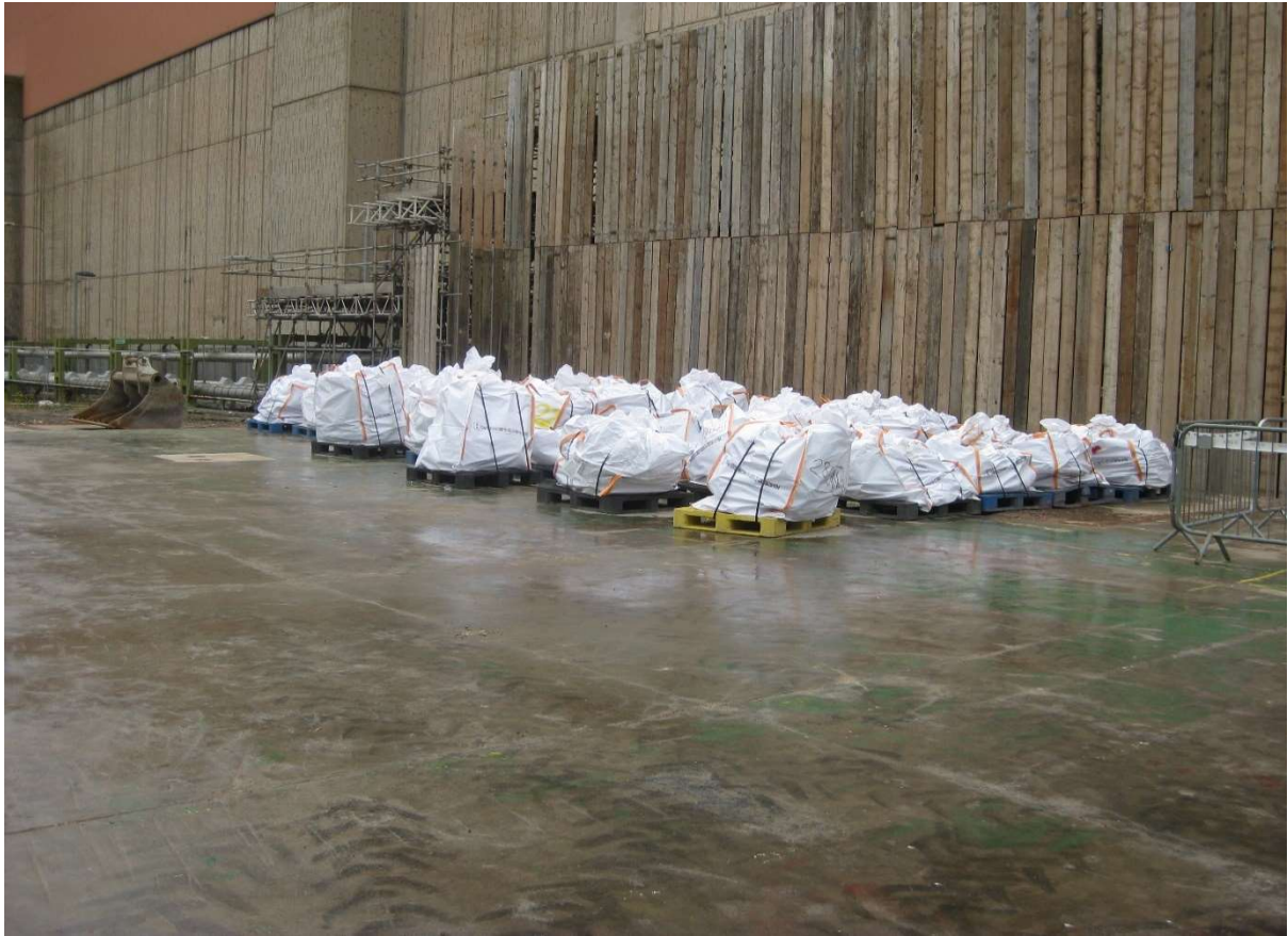
Figure 3: Demolition work completed on Redundant Engineering Workshops waste on base-slab awaiting disposal.
