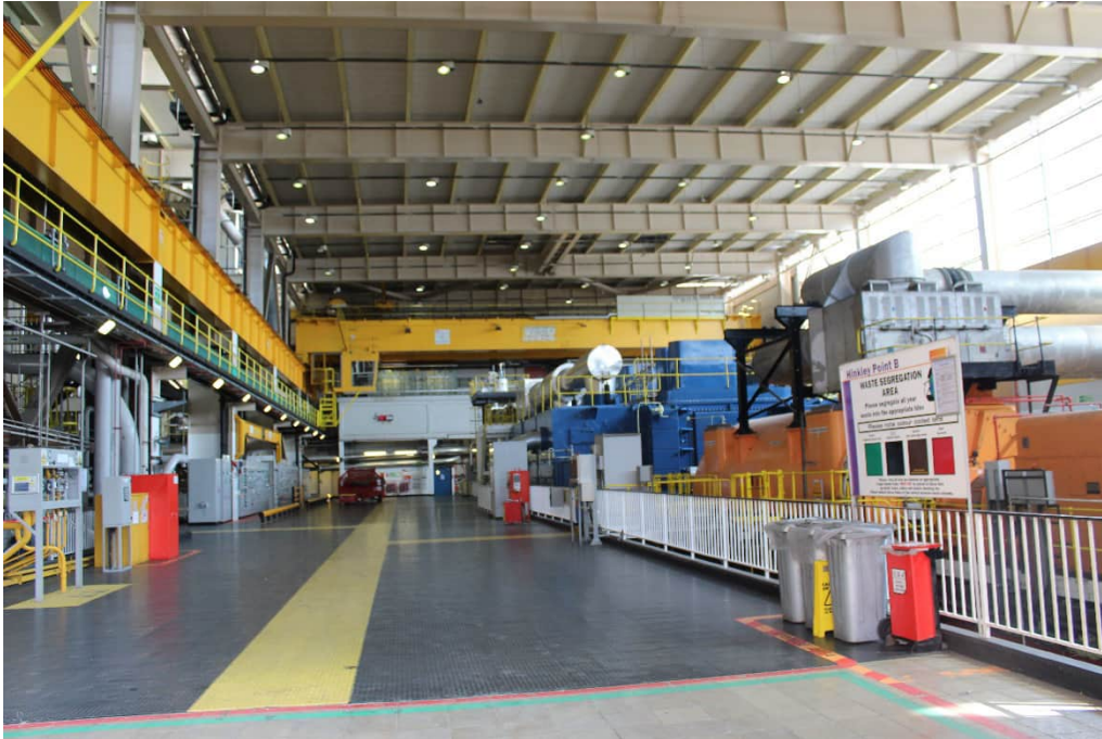
Plate 19. Turbine hall interior.
